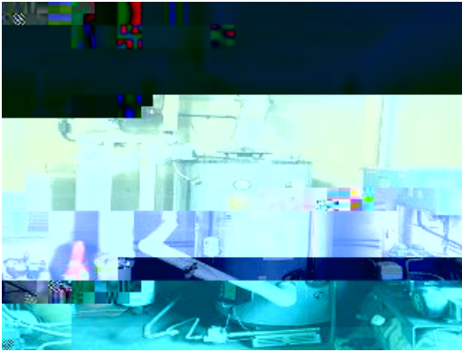
Rusted water heater piping
