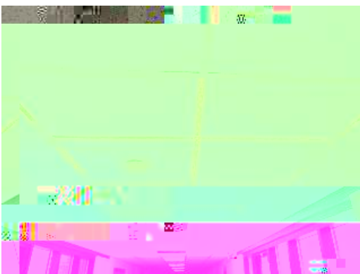
Ceiling grid corroded and damaged.
