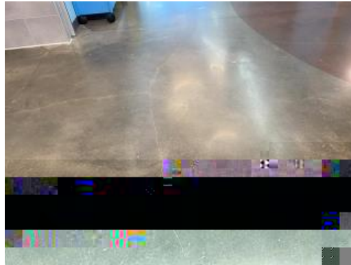
Concrete floor is beginning to crack.
